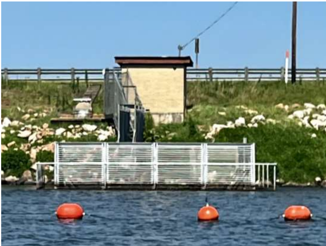
Figure 12: Drop inlet water release structure at Lake Cypress Springs dam
